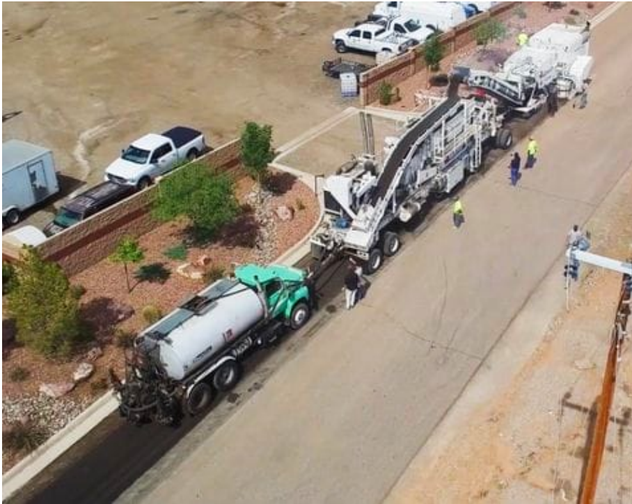
An innovative solution for recycled plastics is hybrid asphalt for building roads
